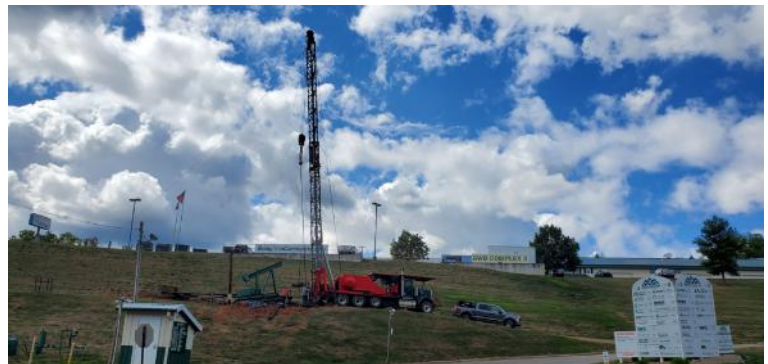
Pictured: Pin Oak service rig servicing one of their wells at the George Broughton's Complex.
